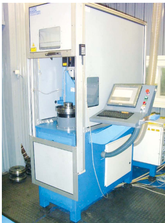
Installation of laser thermal hardening of small-sized parts of BELAZ OJSC
